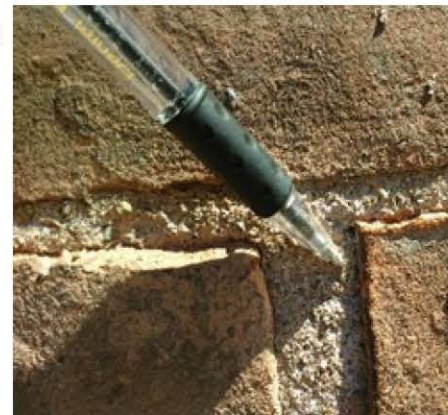
Soft mortar will shed granules of sand when scratched with a key or a pen.
