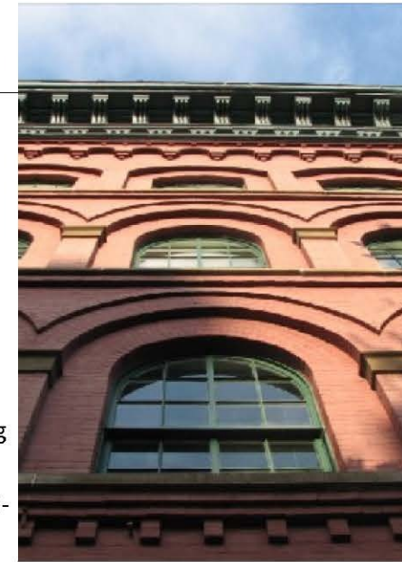
Hard brick, unpainted, is found when the brick pattern and color was a key feature of the design.
