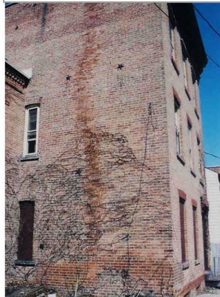
This damage traces the length of a chimney. The temperature differential has eroded the masonry. Repointing is useless without lining the chimney first.
