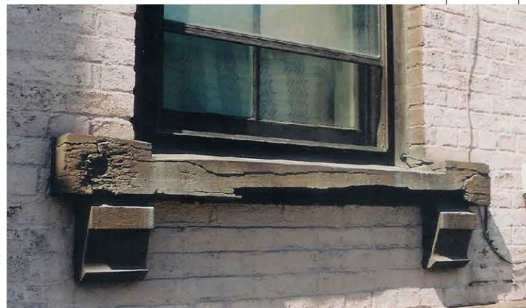
Replacing deteriorated sandstone is an expensive proposition. Very few quarries remain.
