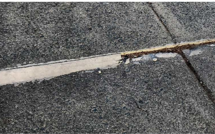
Concrete filler can be used to level uneven surfaces but it won't last long
