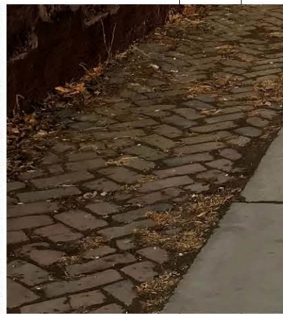
Brick is not a sidewalk material but it makes a nice border
