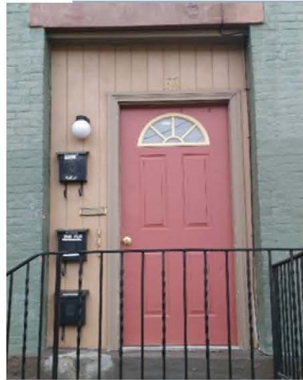
Downsizing a door is inappropriate and not allowed
