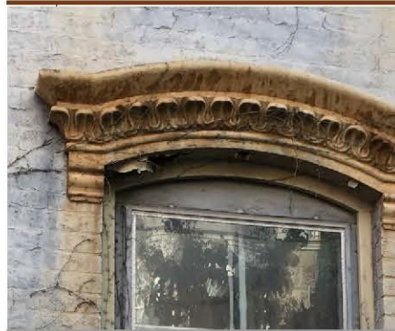
Proper preparation and paint will ensure the longevity of this metal window hood, masonry wall and wood windows.
